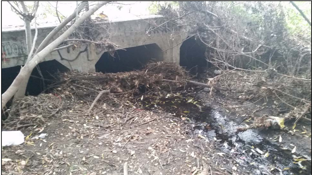
Figure 3. Debris blocking UPRR culvert mouth.
