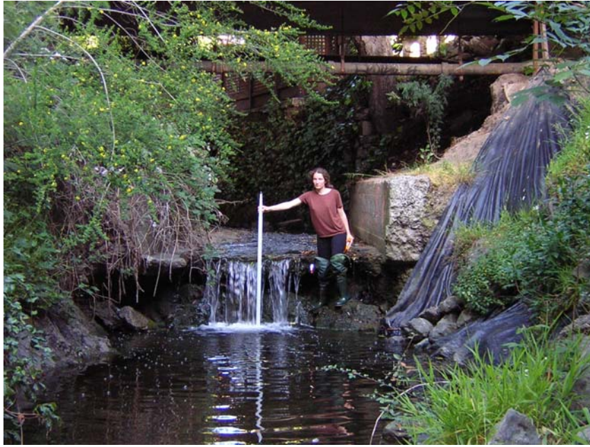
Figure 12. Down-cutting of streambeds below culverts has created most of Codornices Creek's fish barriers
